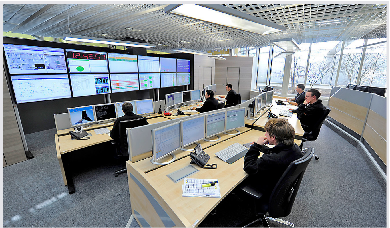
Munich Airport: IT control center of JST
